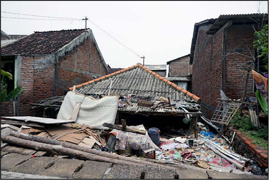
Figure 3: Houses damaged and abandoned due to rob floods and land subsidence in Tambak Lorok fishing village, Semarang.
