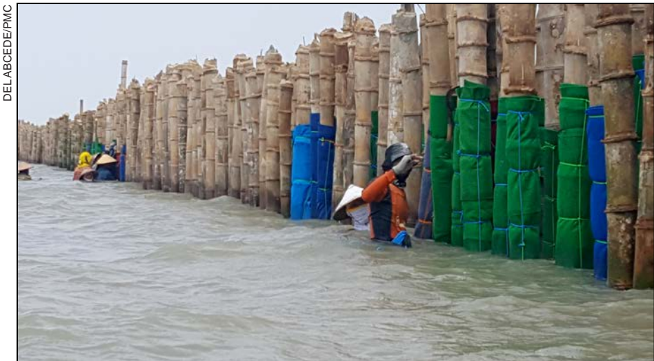
Figure 1: Maintenance workers repair parts of a natural seawall constructed from bamboo near the village of Timbulsloko, Semarang, Indonesia, in November 2017.
