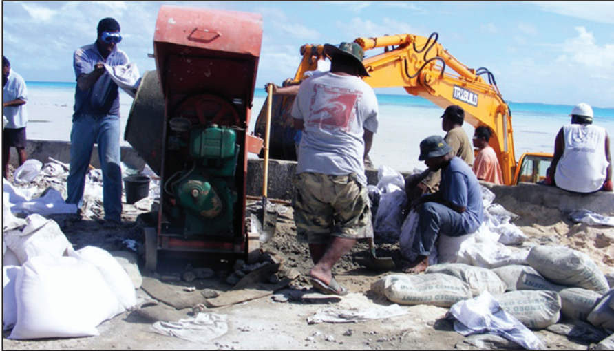
Figure 5: Repair work on the Dai Nippon Causeway Between Betio and Tarawa. Image: Kiribati Independent
