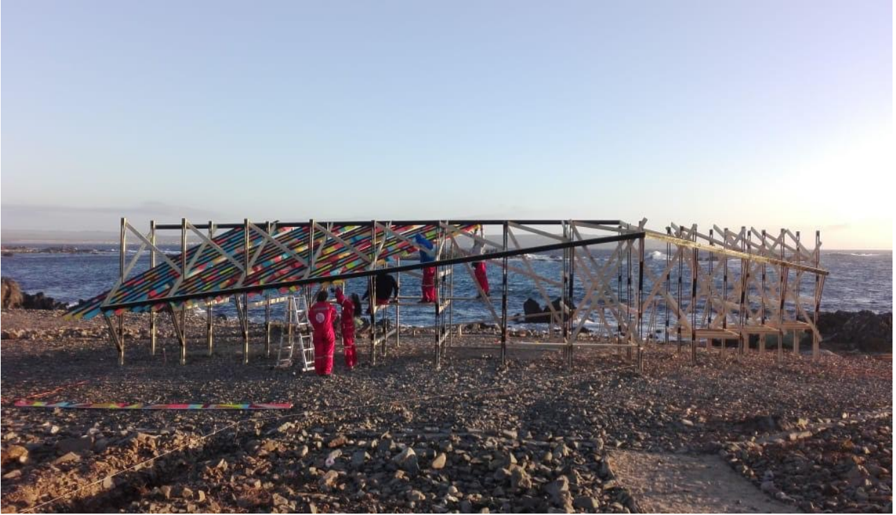
Figure 2. Corredor Litoral. (Coastal Passage) Travesía Caleta Chañaral de Aceituno, 2018. Wooden corridor with a lattice ceiling, integrated seating, and a wind deflector. The latticework is purposefully oriented towards the north, allowing sunlight to filter through and cast coloured patterns within the white interior. Located 20 meters from the highest tide mark, this public work is the collaborative effort of 49 students and 5 professors from the first-year design studios.
