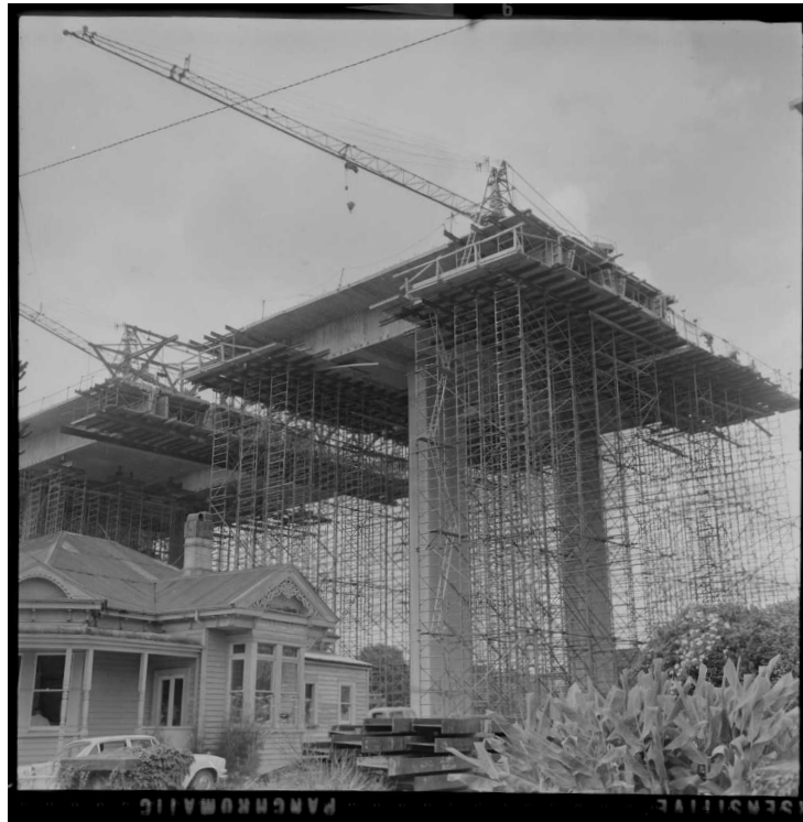
Fig. 1 Whites Aviation (1965). Construction of the southern motorway viaduct, Newmarket. [Photograph, WA-63226-F, Alexander Turnbull Library, Wellington]
