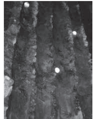
The oozing, dripping and slipping of concrete between the tree trunk formwork” (Photo: author)
